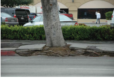
Tree roots uplifting sidewalks
